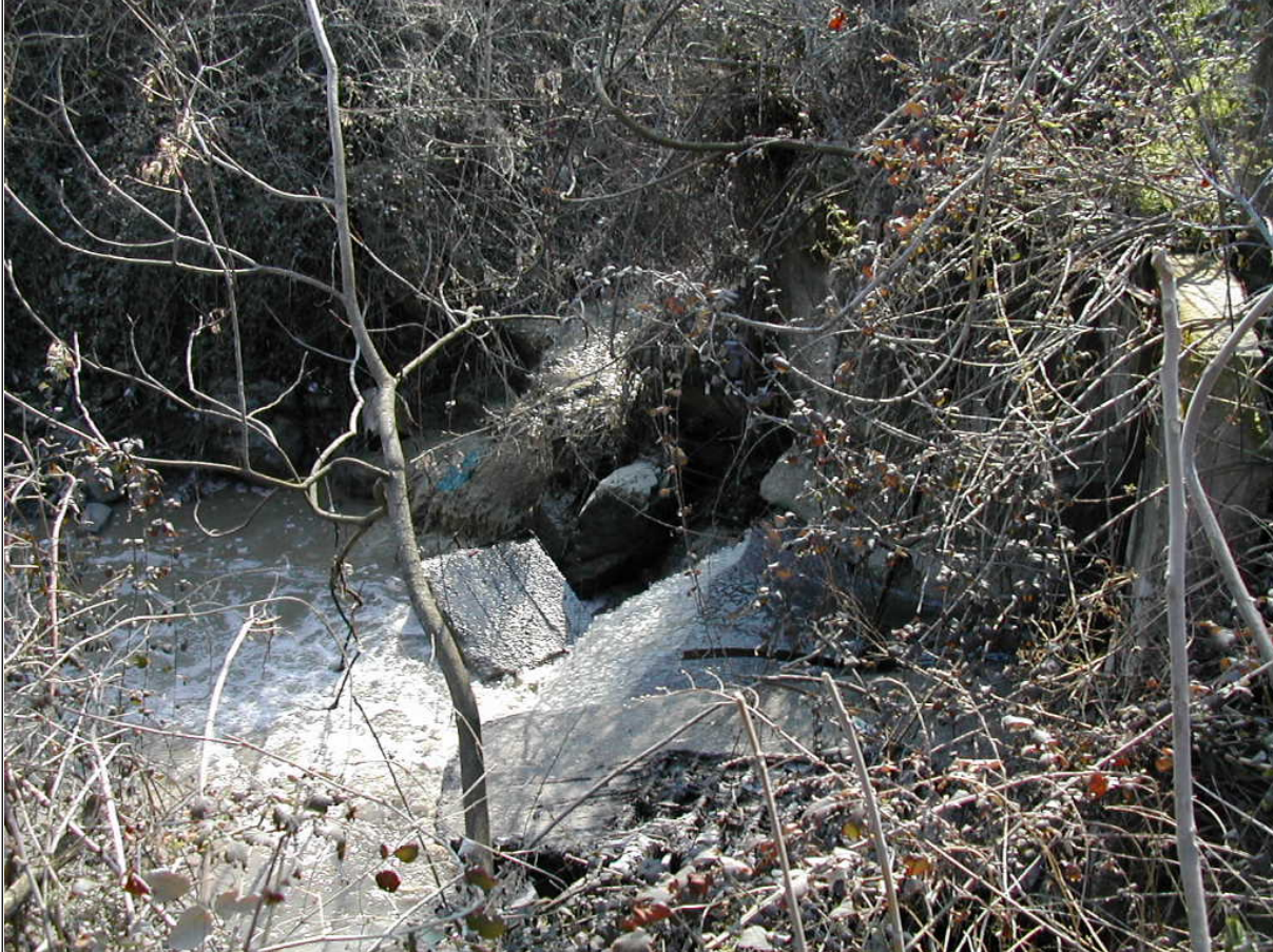
Outflow of the "horse shoe" shaped collector to river Vardar.
